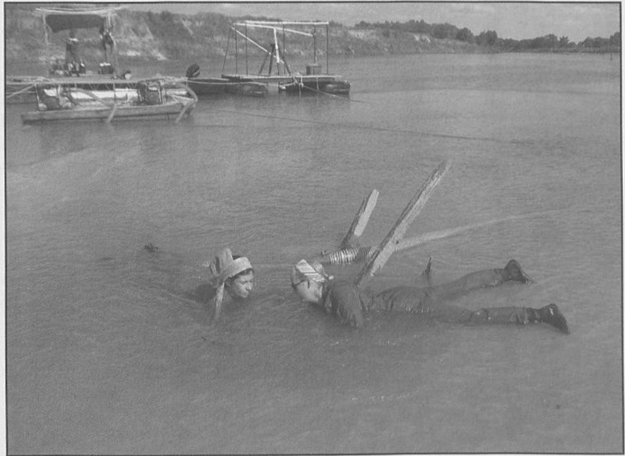
Fig. 12. Maria Cristina Pedroso de Lima (L) and Carrie Sowden commence excavation of the port paddle wheel, the start of a massive trench that would be over 3 meters (10 feet) deep before they finished! Photo: Kevin Crisman
